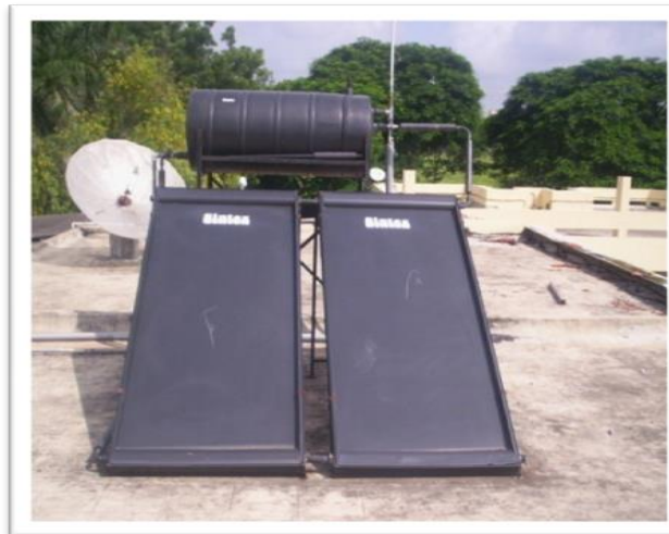
Solar Water Heater
