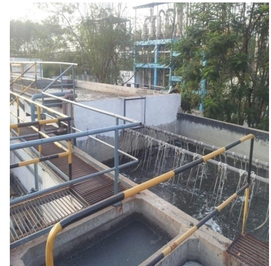
Effluent treatment plant
